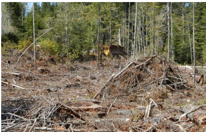
Figure 1. Forest residuals pile and dispersed slash after logging on private forestland near Arcata, CA.
